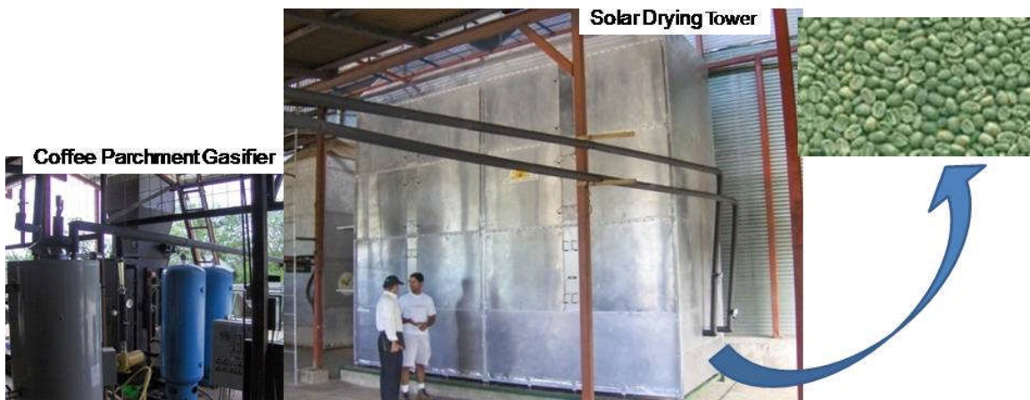
Fig. 2. Solar/Biomass drying systems at Cooperative Montes de Oro, Costa Rica.
